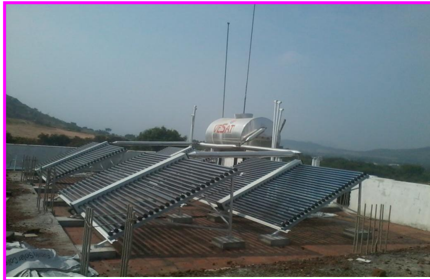
Solar powered water heaters
