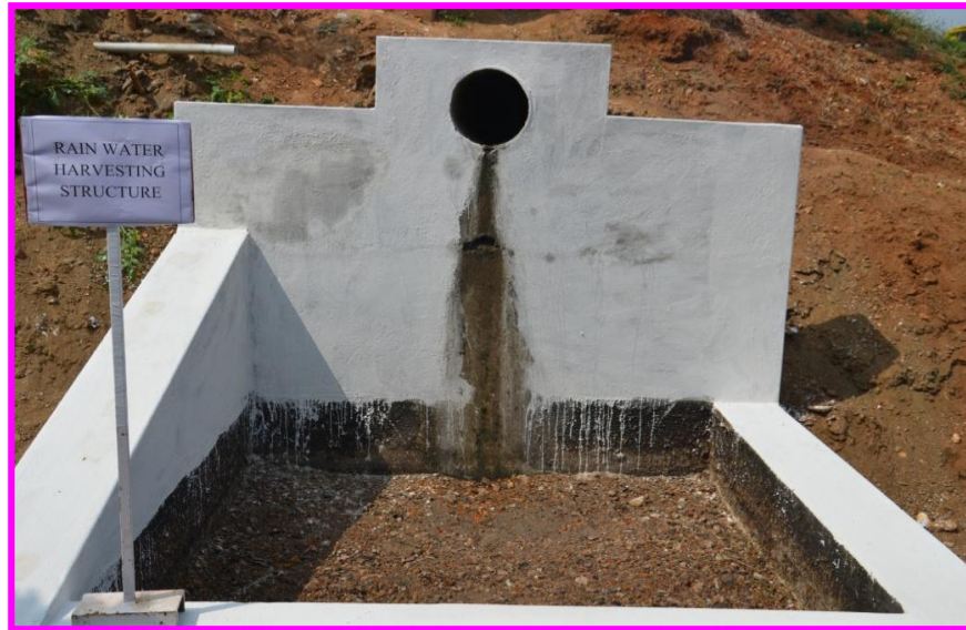
Rain Water Harvesting System
