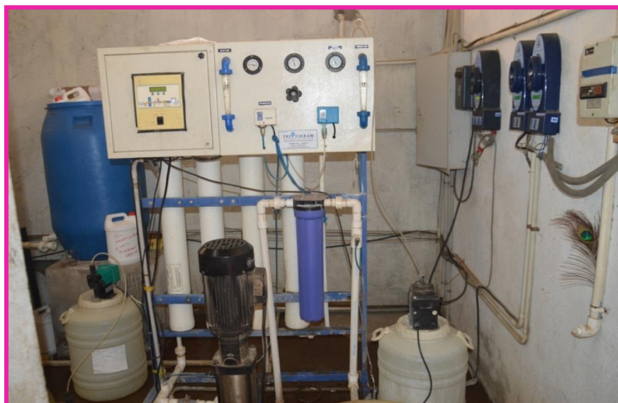
SSEC RO Water Plant
