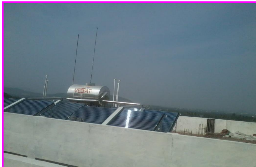
Solar powered water heaters
